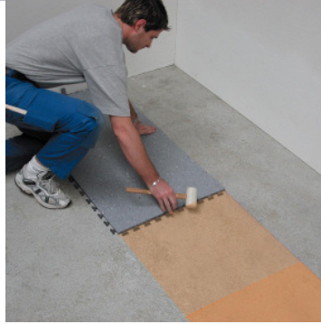
It is important that the second row is installed exactly along the chalk line.
